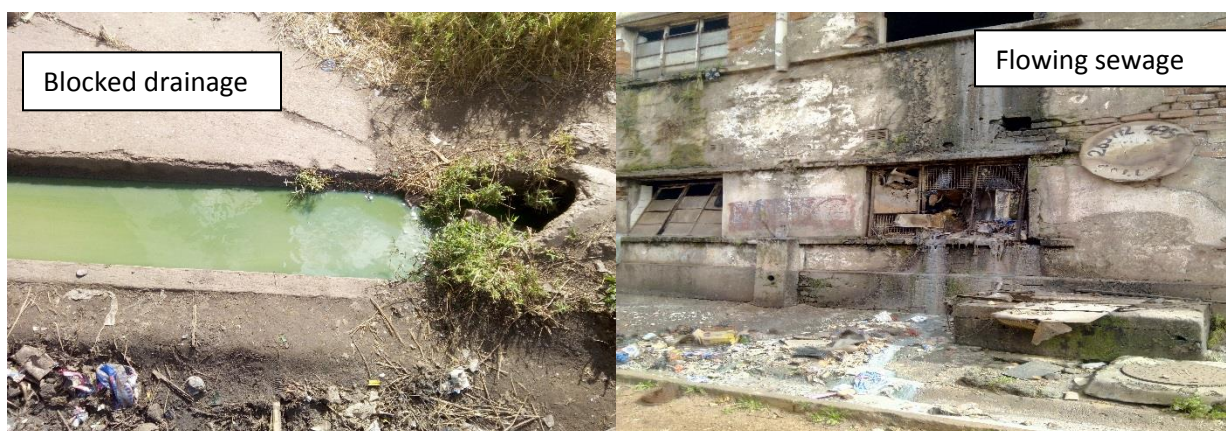
Figure 4.4 Blocked Drainage and Sewer System
