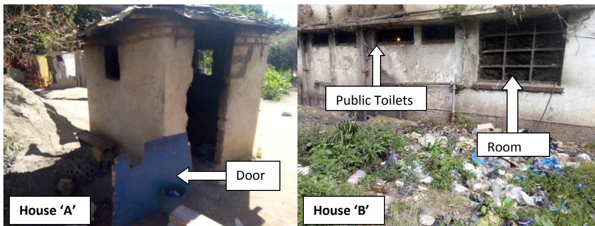
Figure 4.1 Substandard House, Dilapidated Hostel and Toilets
