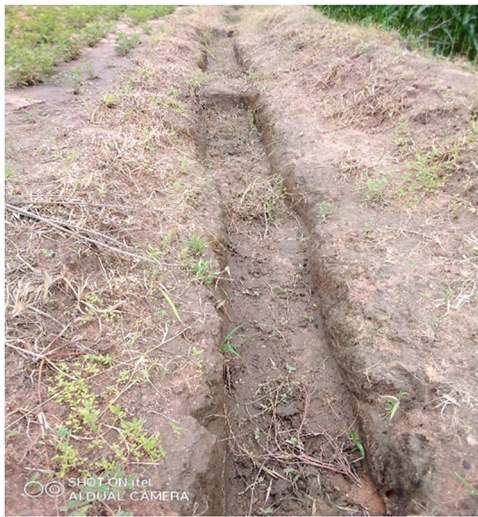
FIGURE 3 Infiltration pits used in Marange, (right)
