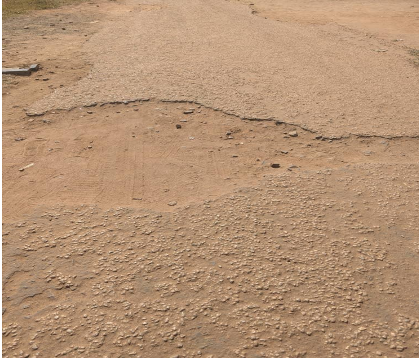
Figure 4.6 the poor state of the Malvern Road observed by the researcher during observations in Waterfalls
